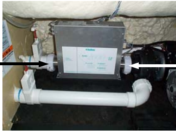
(Figure G) Spa Fittings
